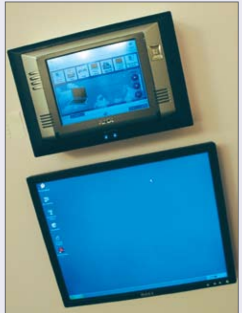
AMX system controls lighting , sound and AV equipment.
